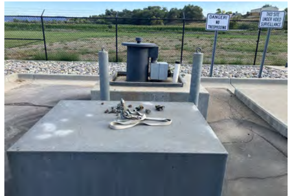
DW8 awaiting final installation
