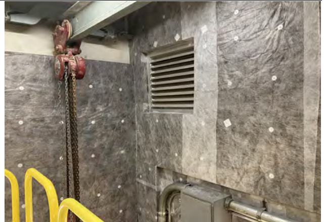
Installed sound dampening acoustical foam
