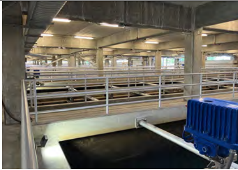
JWTP Filter bay
