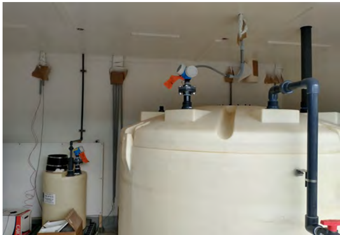
Chemical tanks and piping installed inside new building
