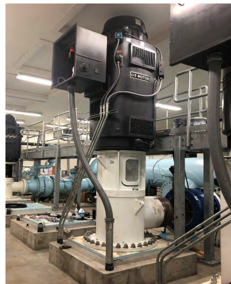
New 1250 HP pump & motor
