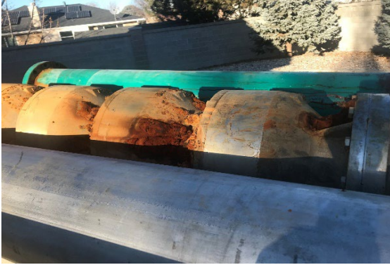
Stainless Steel pump and original well column removed from well showing corrosion
