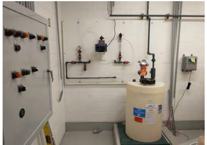
Assembled fluoride day tank feed system
