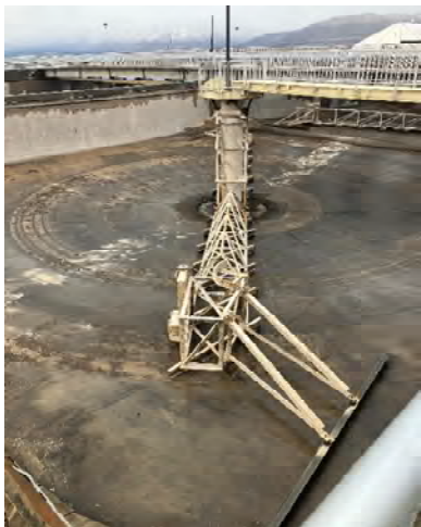
Existing circular clarifier to be replaced with upgraded technology as part of this project
