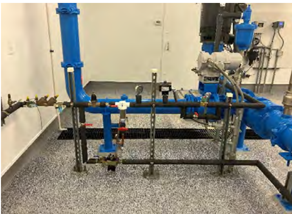
New water "pre-lube" piping (flushes well with city water prior to start up to wet the marine bearings) and reconditioned discharge head/motor awaiting start-up
