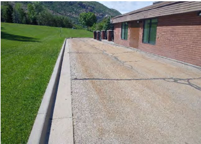
Existing condition of asphalt by ACTIFLO building
