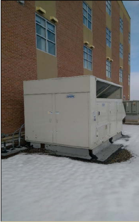
New rooftop air handling unit
