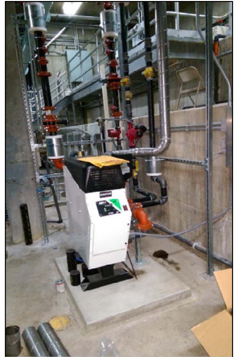
New boiler unit
