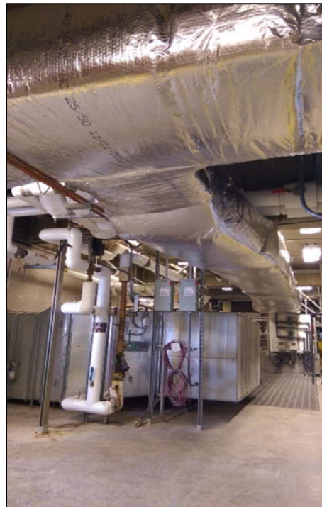
New ductwork to the Laboratory
