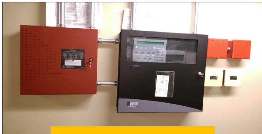
Existing Control Panels (in Filter Gallery)
