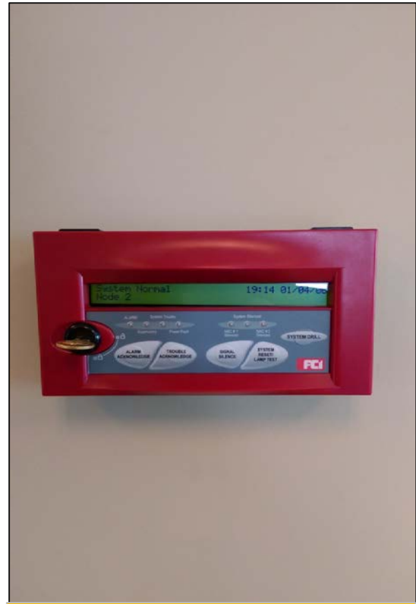
New Control Panel (behind the Operators Room)
