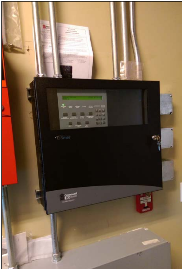
New Enunciator Panel (in Control Center)
