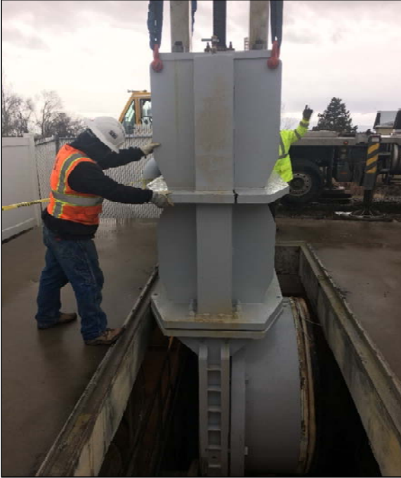
The damaged gate valve being removed from Station 308 on the Jordan Aqueduct Reach 4
