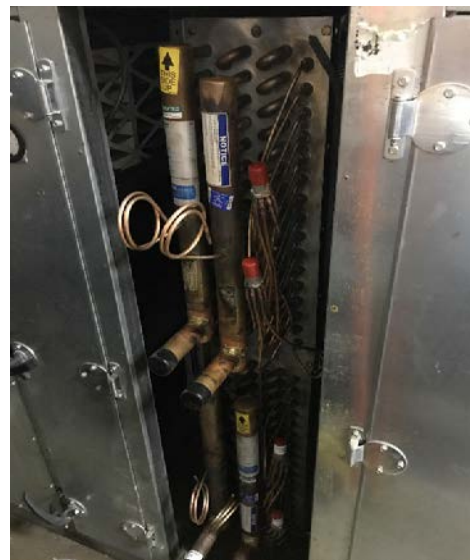
New Coils in Air Handler Unit
