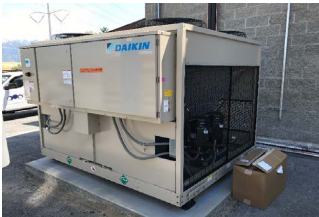
New Condensing Unit
