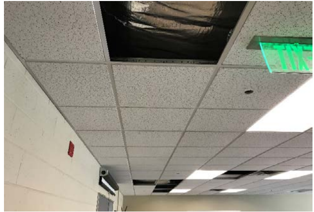
Ceiling Duct and Insulation
