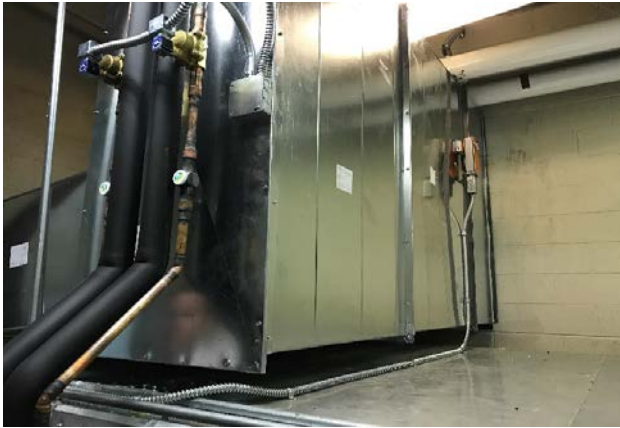
Mechanical Room Completed Ductwork
