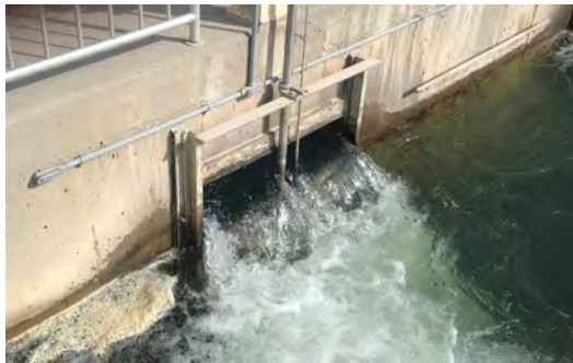
Raw water entering flocculation basin
