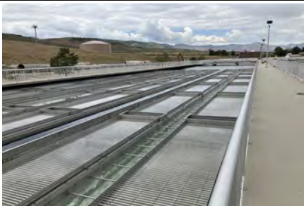
JWVTP Basin 6 on-line producing high-quality settled water
