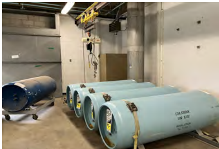
Existing gaseous chlorine system
