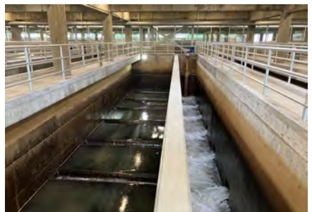
JWTP Filter undergoing backwash
