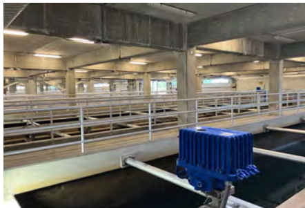
JWTP Filter bay
