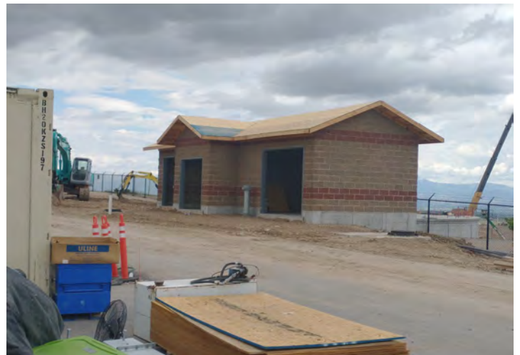
New chemical feed building
