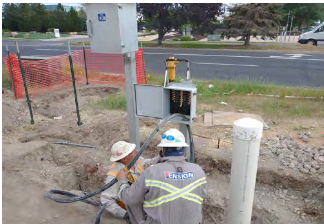
Contractor working on installing anode junction box between well bed and rectifier
