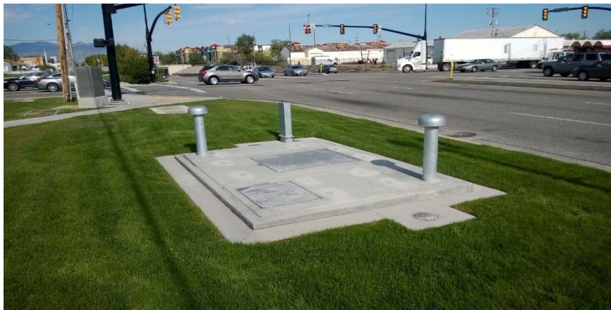
Main Street 4500 South new concrete vault
