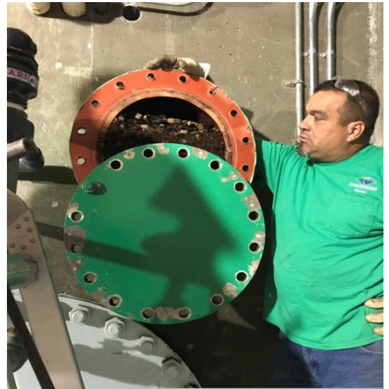
Corrosion by-product from unlined steel piping.
