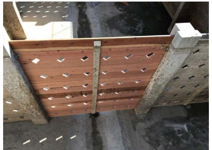
New Redwood baffles.
