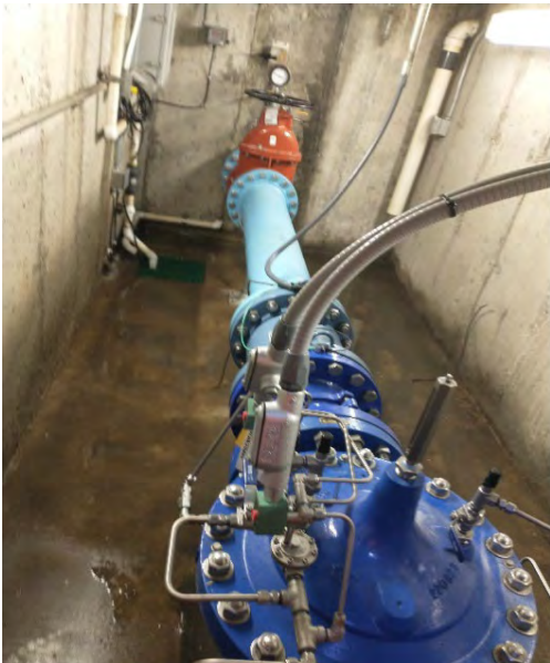
New pipeline, meter, and valves
