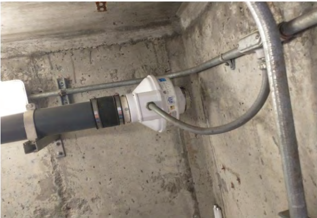
New installed ventilation fan
