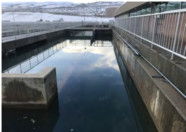
JWTP Distribution box in operation after raising of hydraulic grade line
