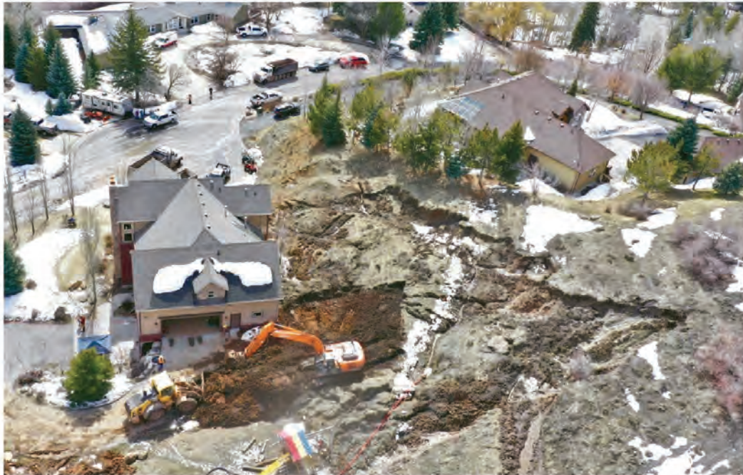
Crews work to clean up and stabilize a hillside Monday after mud came sliding down a hill in this Morgan neighborhood in northern Utah.
