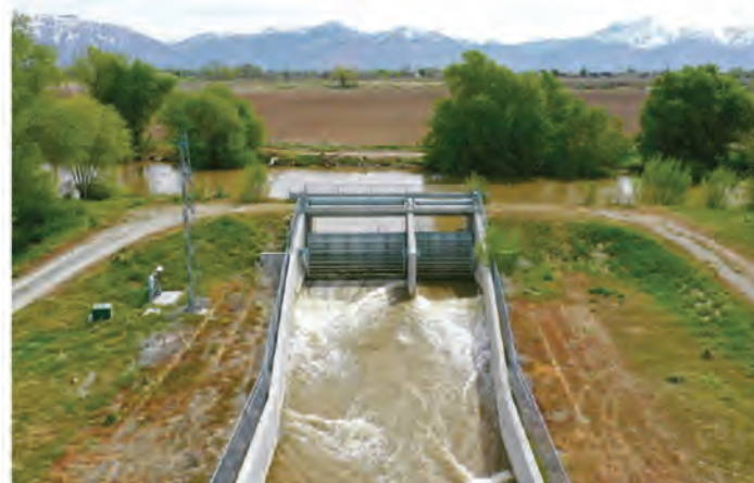
The Little Weber River Cutoff Channel Project, a $26 million project that diverts water from the Weber River to the Ogden Bay Waterfowl Management Area and the Great Salt Lake, is pictured in Warren, Weber County, on May 10. Kristin Murphy, Deseret News
