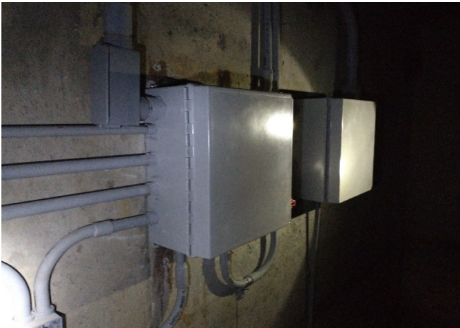
New electrical boxes in vault.
