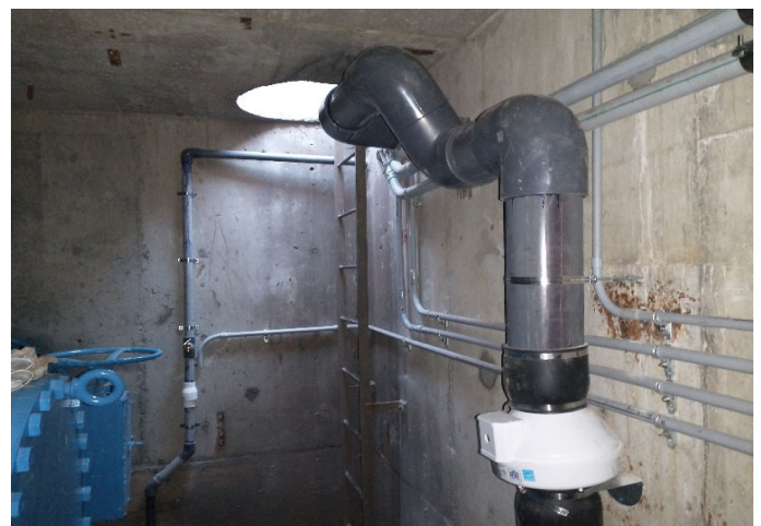
New ventiation fan and line in vault.
