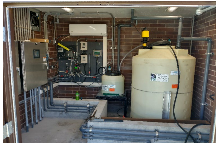
9800 S 2300 E interior piping and tanks
