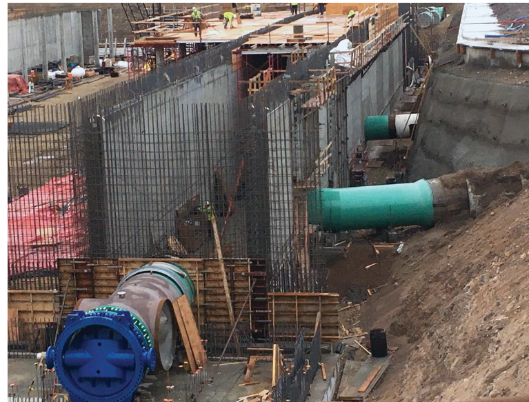
Opposite page: 78-inch finished water connection from new 12.5 MG reservoir at JWTP. Photo by David McLean.
