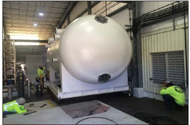
Setting of pressure vessel
