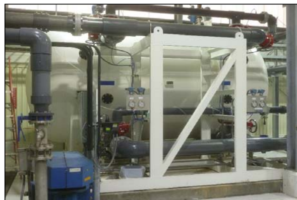
Installed and operating manganese pressure filter
