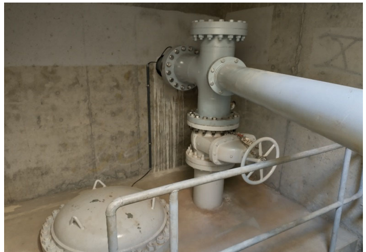
New Vault Piping at Pleasant Grove Location
