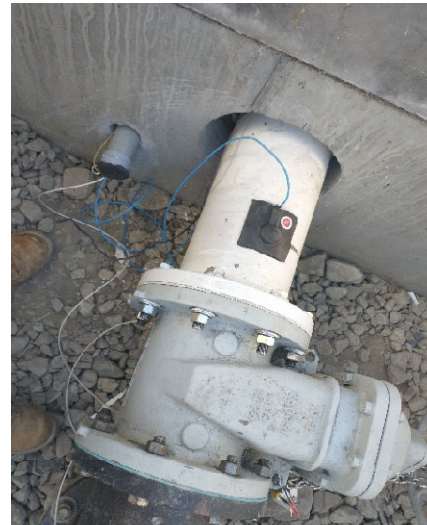
Connection to PRA with cathodic monitoring wires at Pleasant Grove Location
