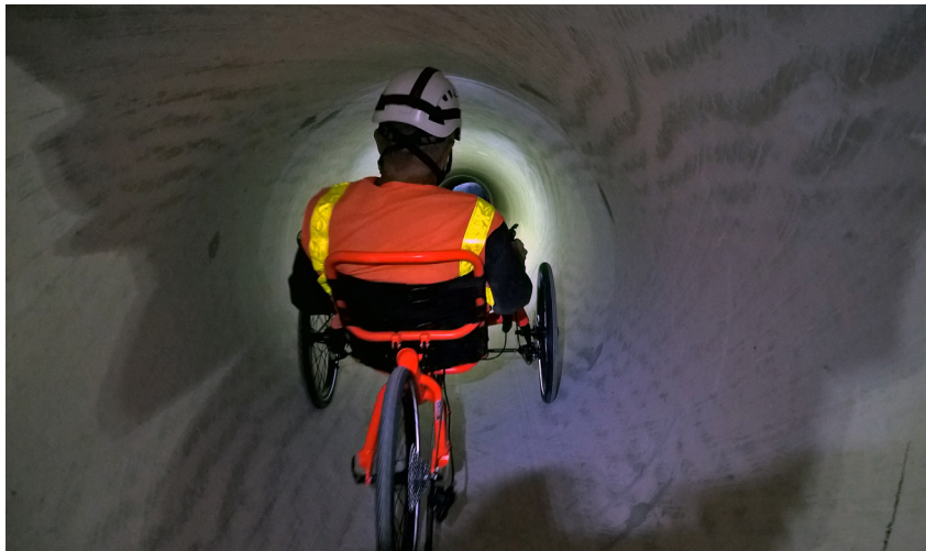
Left photo: Inspection of the completed Central Pipeline Project interior. Right photo: Installation of the 10200 S. Capacity Improvements Project under Bangarter Highway.
