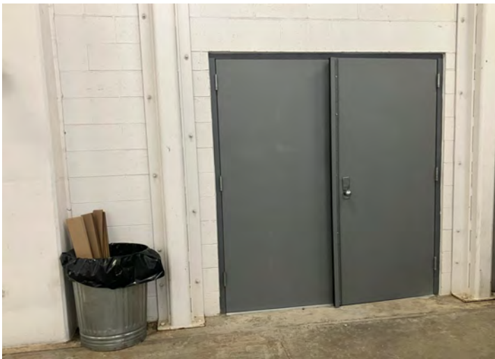
Installed high-performance sound attenuating door
