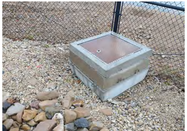
The electrical pull box raised above the flood level
