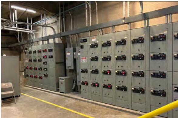
30 year old motor control center scheduled for replacement with this project
