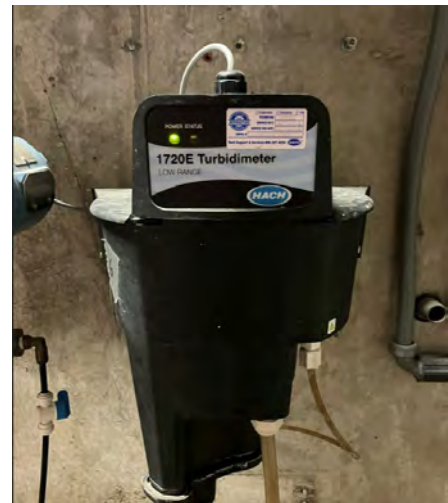
Turbidimeter providing operators measurement of the water quality from the plate settlers
