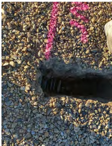
Potholing the edge of the reservoir and the conduits running along the side
