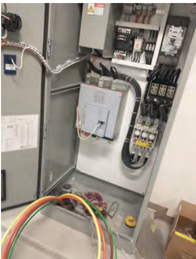
The new reduced voltage soft start
