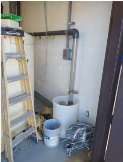
Chemical tank overflow piping and containment
