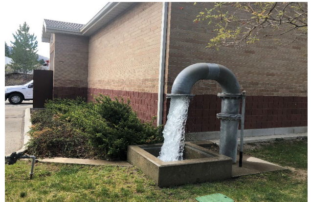
Pump to waste during well start-up.
