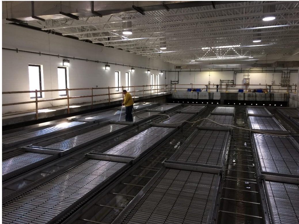
Figure 4.10 Routine Plate Cleaning from Above
