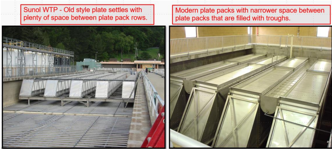
Figure 4.6 Old-style and Modern Plate Pack Installations
