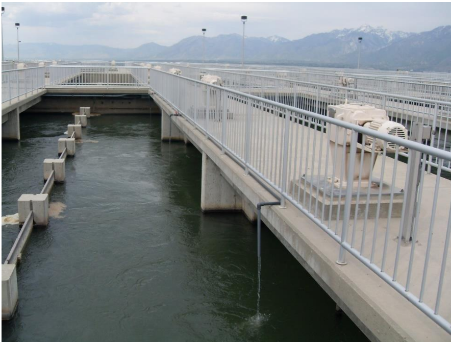
Figure 3.7 Temporary Flocculant Aid Piping at JWVTP (circa year 2009)
