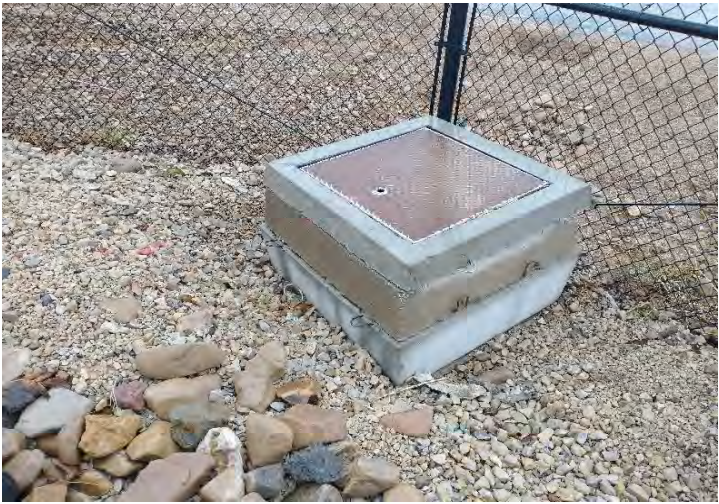
Electrical Box raised to prevent flooding inside
