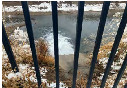
Pump to waste disposal to Utah and Salt Lake Canal
