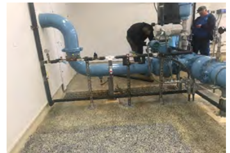
Contractor personnel completing final adjustments prior to start up
