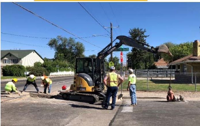
Removing gate valve to abandon the existing cast iron pipe from the distribution system.
