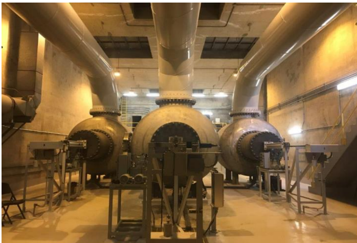
Sleeve Valves at JA-4 Flow Control Structure
