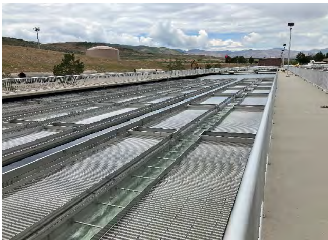
Operating plate settlers
