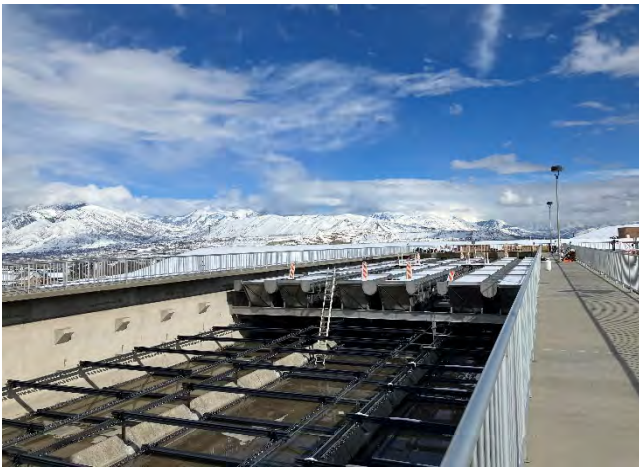
Installed sludge collection equipment and plate packs
