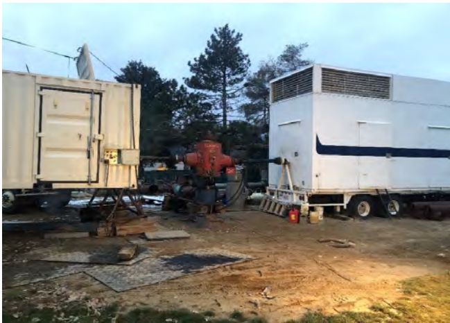
Dual-drive engines for Etienne well pump test
