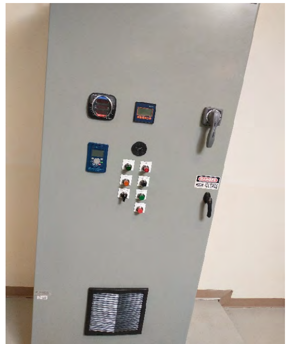
New Electrical Soft Start
