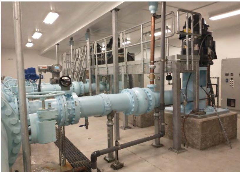
Completed pump, motor, valves, and piping
