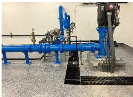
Deep Well 7 internal piping
