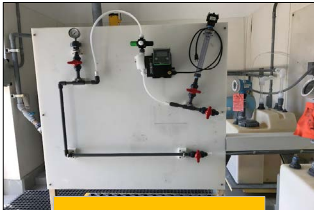
New chemical pump panel
