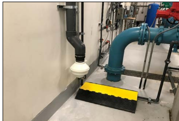
New safety ramp and fan at 1453 East 9400 South
