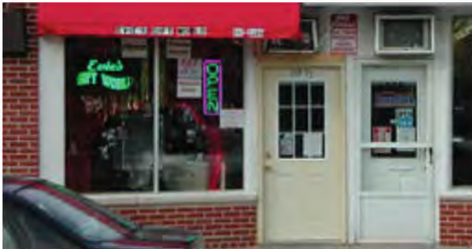
Prohibited: Residential Grade Doors on Commercial Buildings.
