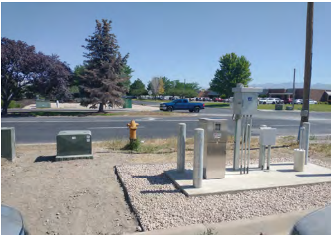
The completed rectifier, well pad, and power transformer
