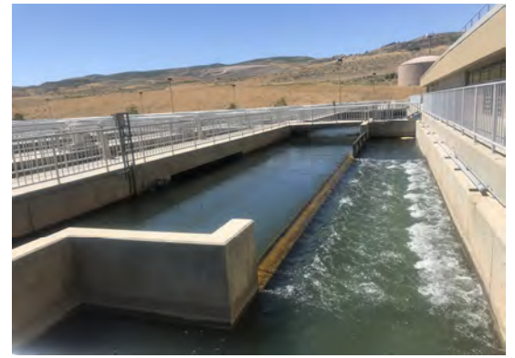
JWWT Distribution Box to be upgraded for improved fluid distribution as part of this project
