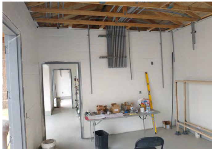
Conduits in the new fluoride room
