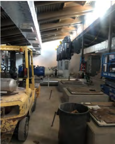
Pumps and motors are in place at the new pump station
