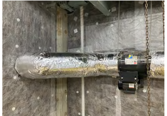
Welding room fan with acoustically insulated ducting
