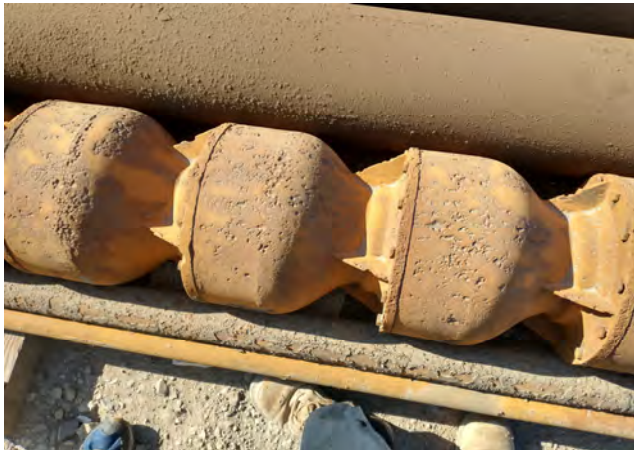
The pump bowls showing significant corrosion and pitting
