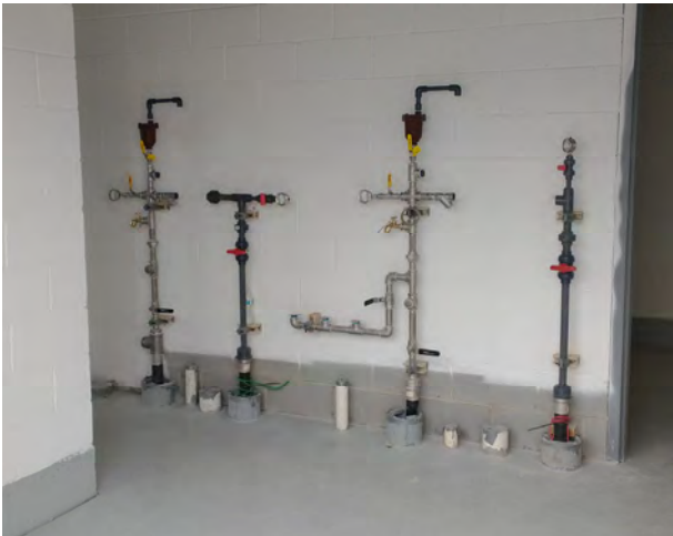
Piping in new building for chemical analysis and injection
