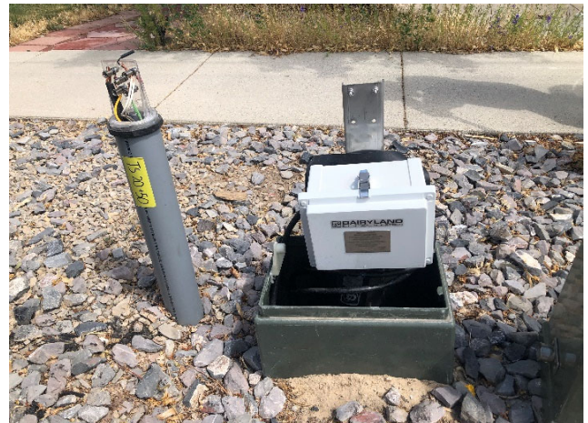
DC blocker and test station
