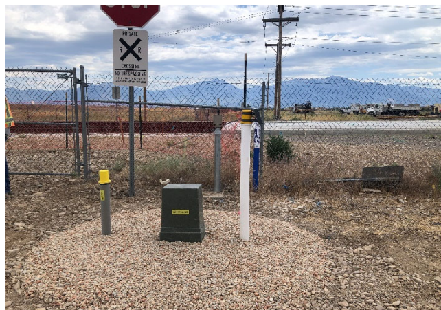
MetriCorr monitoring equipment and DC blocker
