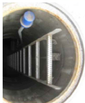
MH, Ladder, Cathodic
