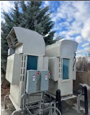
South Education Center Building Heat Pumps
