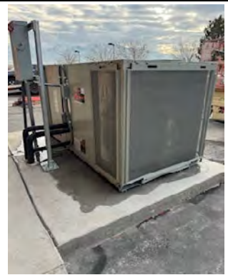
SWGWTP South Heat pump
