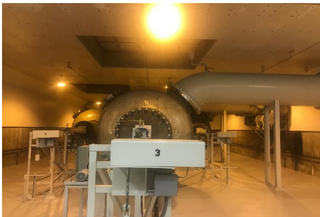
Sleeve Valves at JA-2 Flow Control Structure
