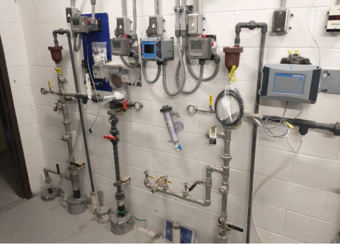
Monitoring Equipment in new Chemical Building
