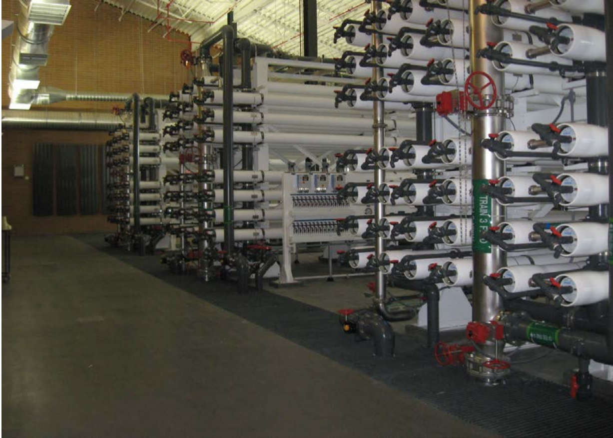
RO Membrane Systems
