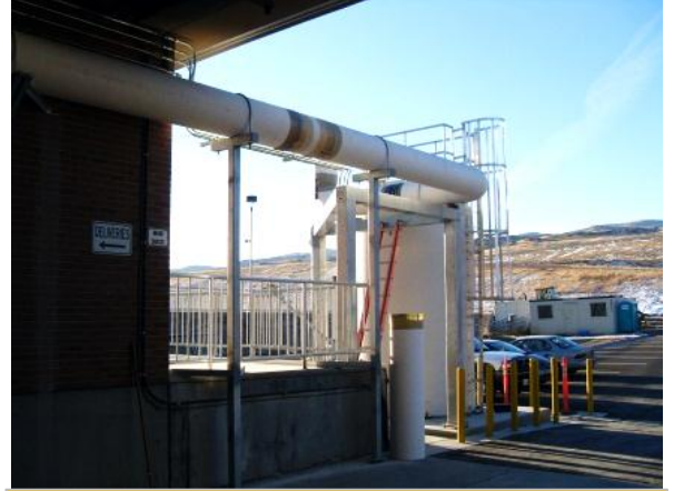
Replacement chlorine scrubber unit
