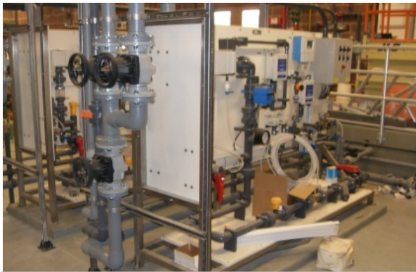
2,500 pound per day CL02 generator
