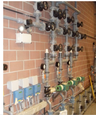
CL02 solution distribution
