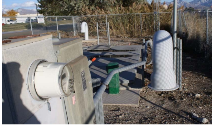
2100 South 3730 West vault
