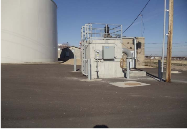
New air gap structure 4700 South 6000 West Reservoir site
