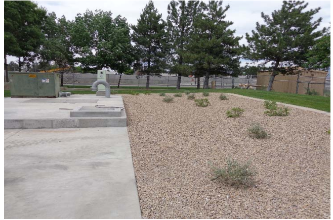
2100 South 3737 West vault
