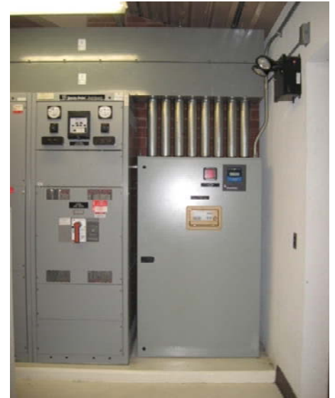
Completed switch gear
