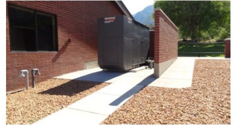
Close-up of completed 300 kW generator installation
