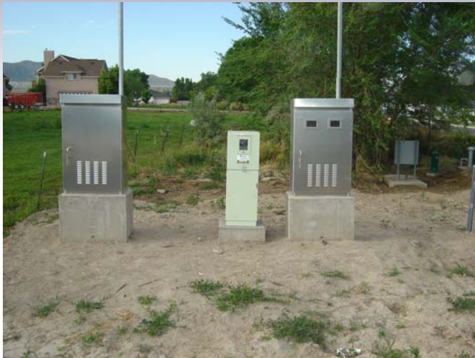
South Jordan City meter station at 700 West 11400 South
