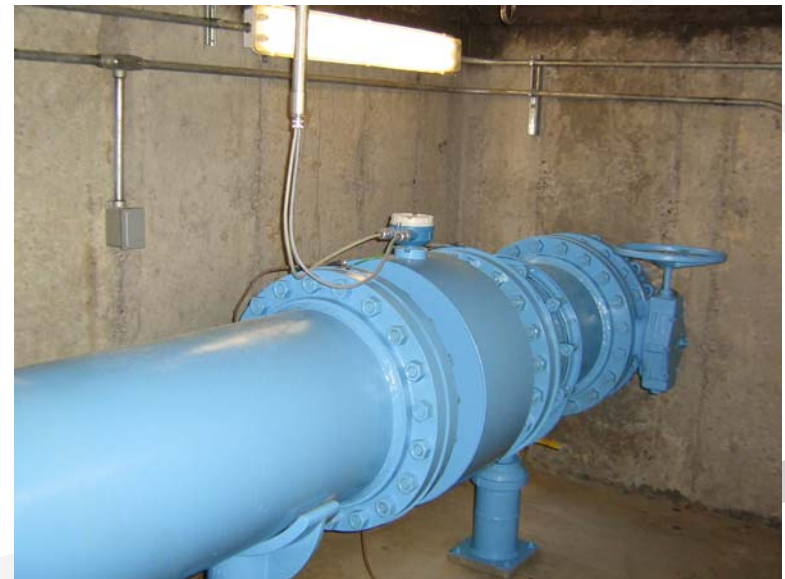
Completed meter station vault interior at 5200 West 6200 South
