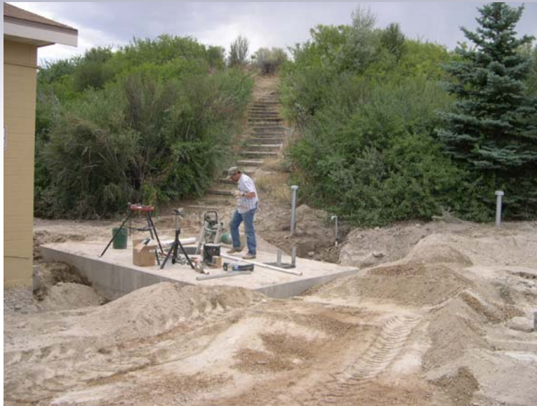
Kearns Improvement District master meter at 5200 West 6200 South
