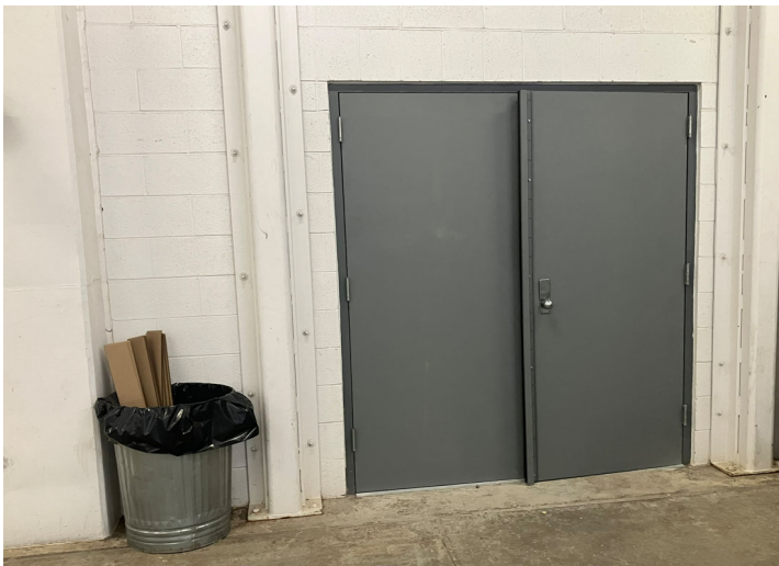
Installed high-performance sound attenuating door
