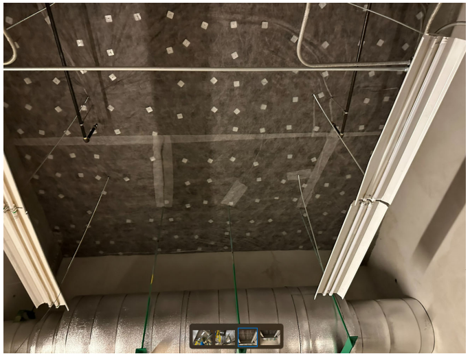
8" of Sound attenuating ceiling foam between blowers and lab
