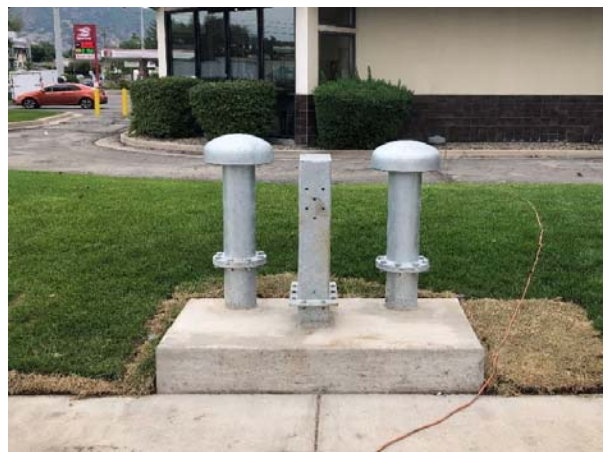
Mushroom vault vents and air-vac cover.
