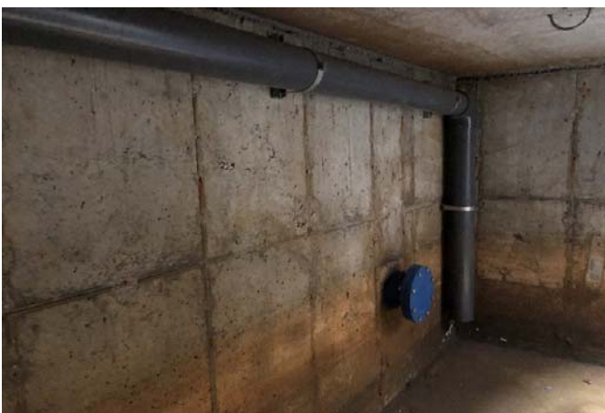
Passive vault vent piping.
