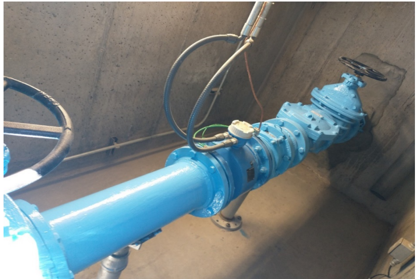
New flow meter installed with new valves, piping, and stands in the vault
