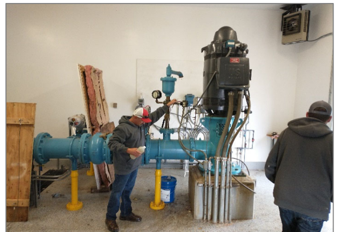
Reassembled pump operating
