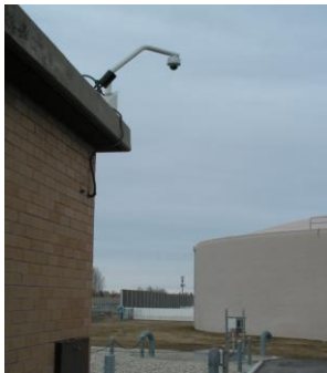
New cameras installed at 3600 West 10200 South
