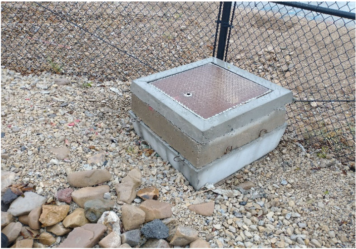
Electrical Box raised to prevent flooding inside
