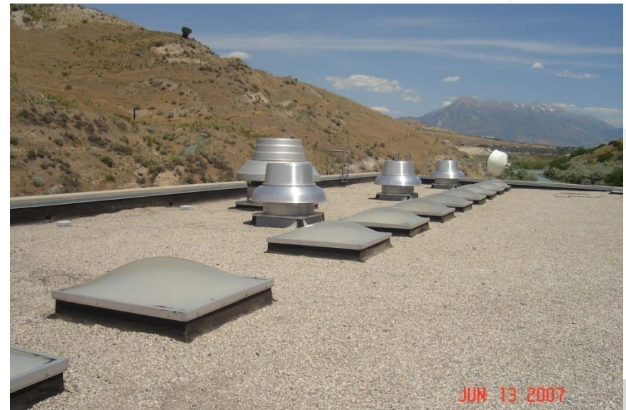
After Four new 15,000 CFM roof mounted exhaust blowers
