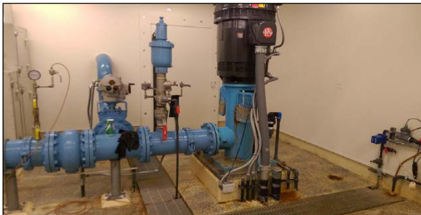
New pump installed and operating DW7
