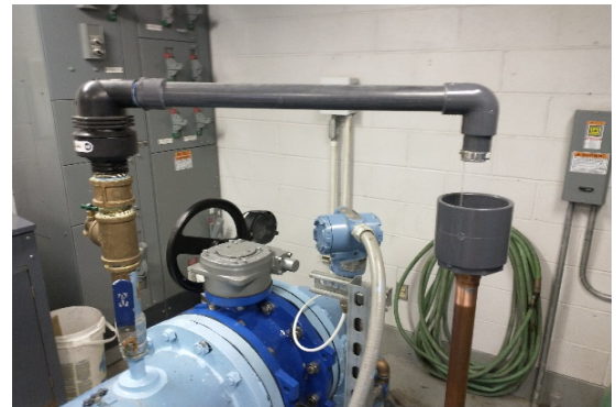
Modified air vac line
