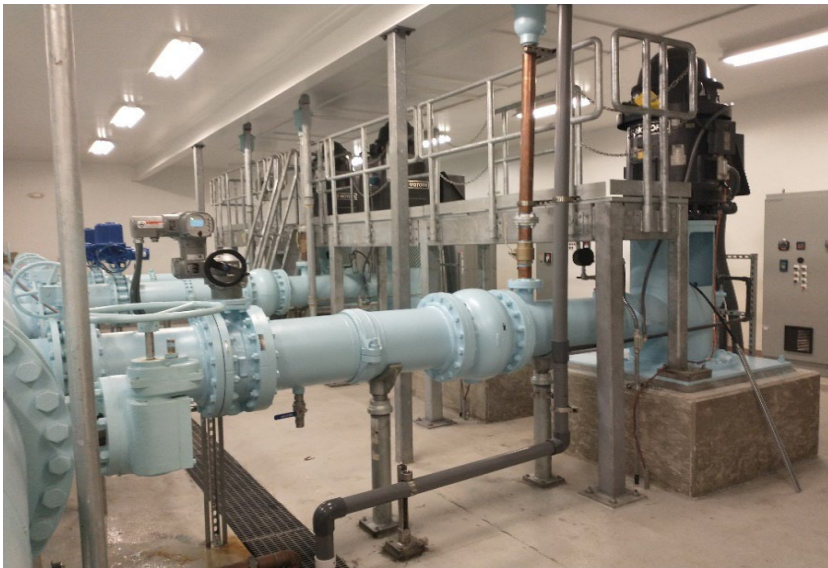
Completed pump, motor, valves, and piping
