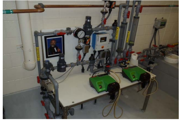
Chlorine Feed Pumps
