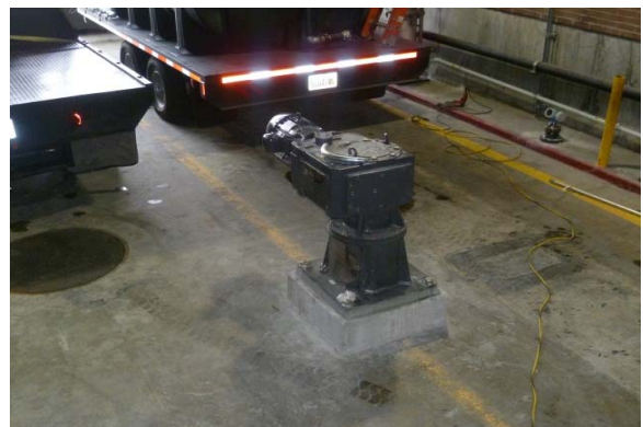
JVWTP PAC Mixer
