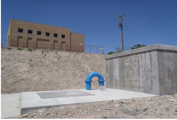
Chlorine Booster Facility & Chlorine Injection Vault
