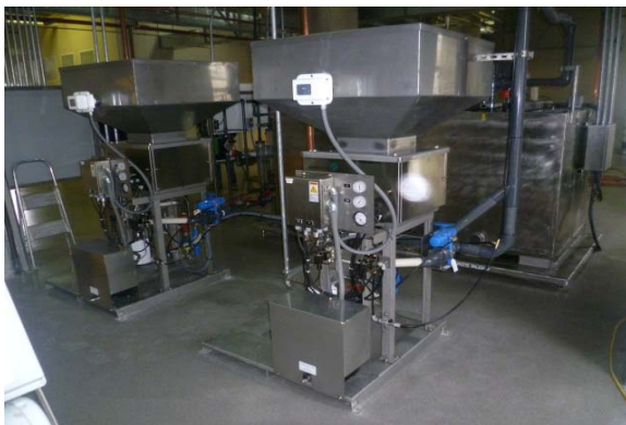
JVWTP PEA Polymer Mixing and Feed System
