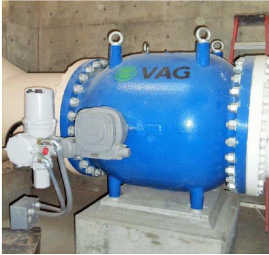
Plunger valve installed at the Jordan Narrows
