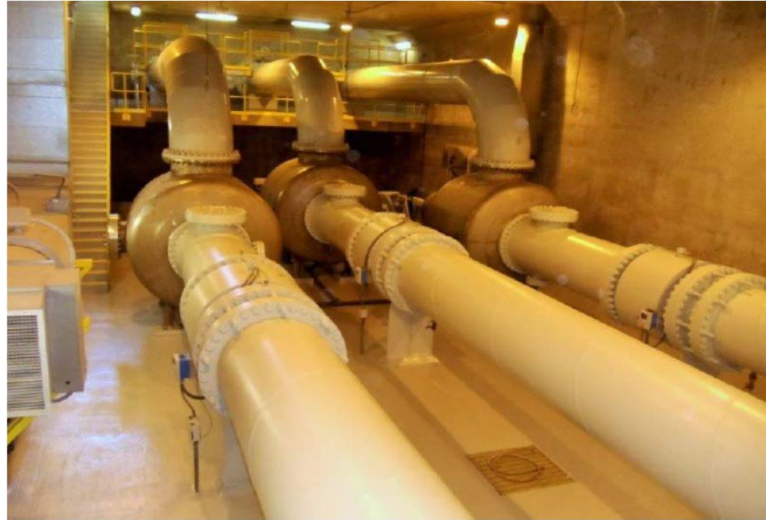
New meters in the Sleeve Valve Vault
