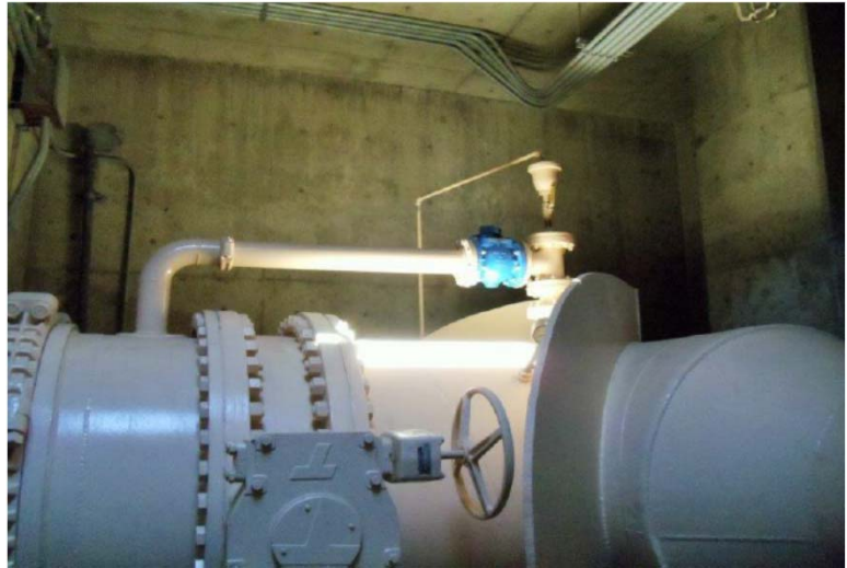
New bypass line at Jordan Narrows
