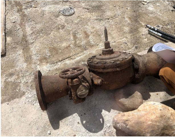
Old Gordon Lane pressure reducing valve assembly
